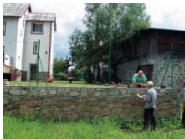
Individual activity – flood wall, Gorzanow (Poland)
